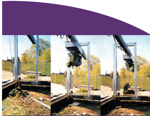
The Bosker Overhead Trashrake operating fully automatically under heavy debris conditions
